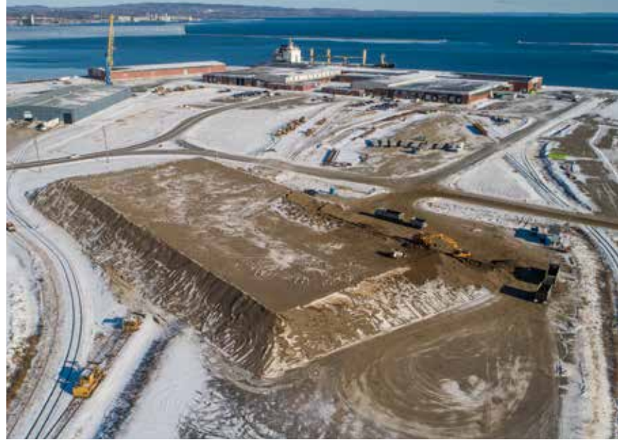
The pre-load for a new 50,000 sq. ft. heated transit shed nears completion in November 2018. Construction on the building will commence in summer 2019
